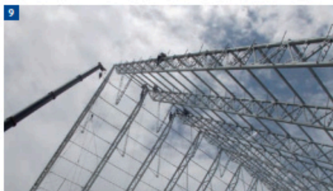
Sugar Warehouse, Santos, Brazil (Foto 9: Photo courtesy of ICZ-Instituto de Maetais Nao Ferrosas)
